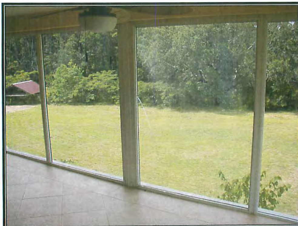
View of the backyard and the Perdido River from the Florida Room (2 nd Level), note the cracked glass window
