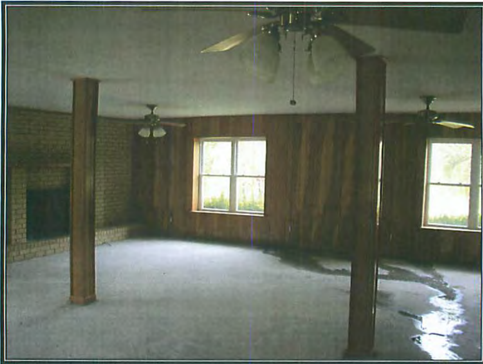
View of a family room (1 st Floor), according to Mr. English the water on the floor is more than likely coming from a clogged air conditioning line
